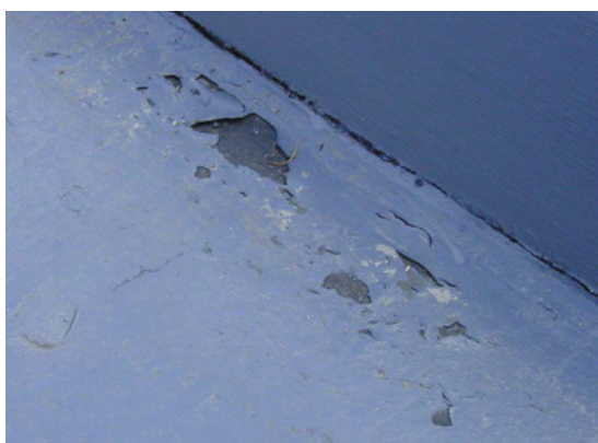
Fig. 12 Deterioration of conductive paint due to rain water pooling
