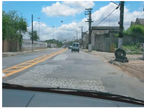
(b) Mixture of Brick road and asphalt paving with high waviness
