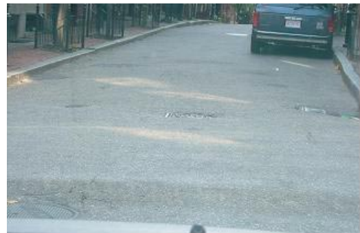
(b) Many indentations on road surface by manholes
