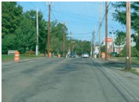
(a) Slightly distorted asphalt road
