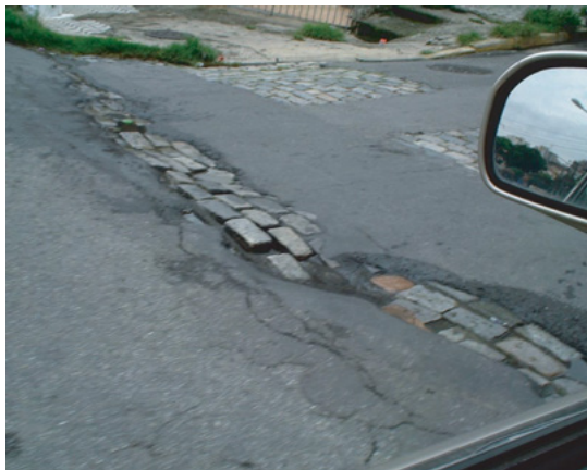
Example of road surface where squal occurs in irregular section
