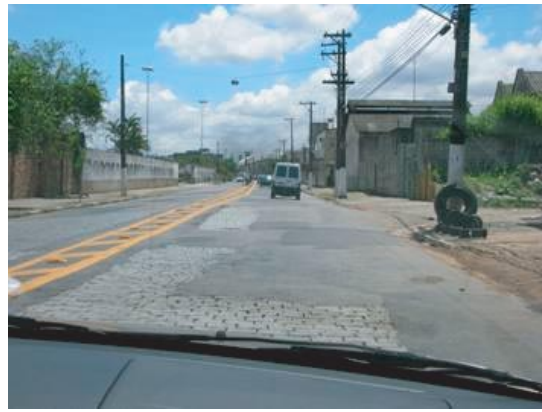
(b) Mixture of Brick road and asphalt paving with high waviness
