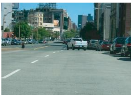
(c) Undulating road surface
