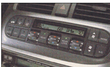
Fig. 8 Heating control switches
