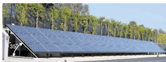
Fig. 7 External view of photovoltaic modules
