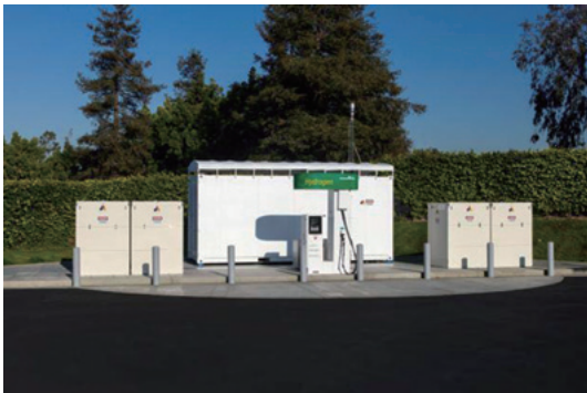
Fig. 7 Hydrogen refueling station at which MC-Formula was applied
