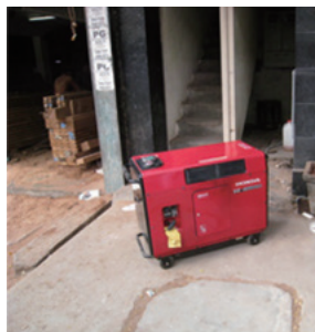
Fig. 1 Example of generator usage in India
