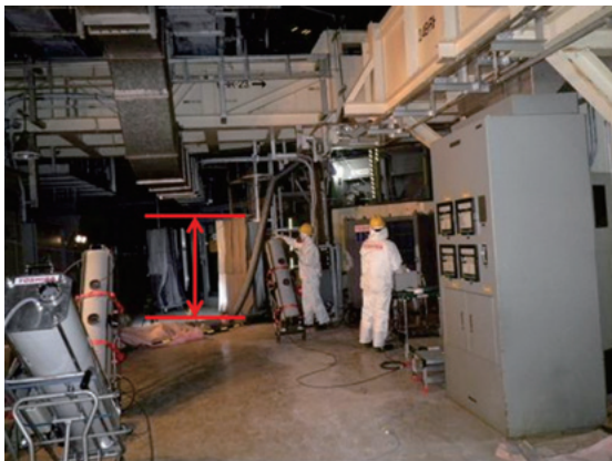
Fig. 4 Inside reactor building (Image provided by TEPCO)
