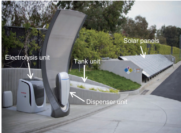
Fig. 1 External view of Solar Hydrogen Station (SHS2)
