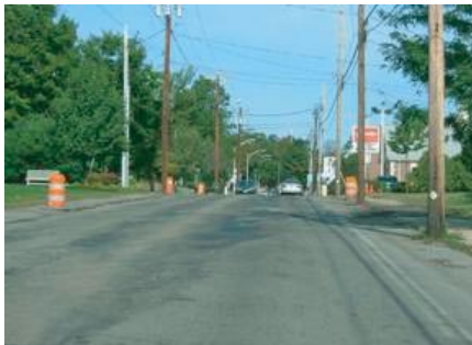
(a) Slightly distorted asphalt road
