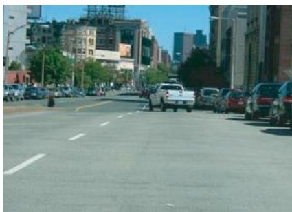
(c) Undulating road surface
