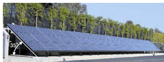
Fig. 7 External view of photovoltaic modules
