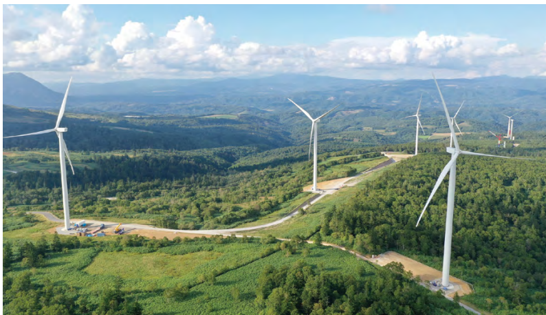
Rusutsu Wind Power Plant (Rusutsu Wind LLC) (Japan)
