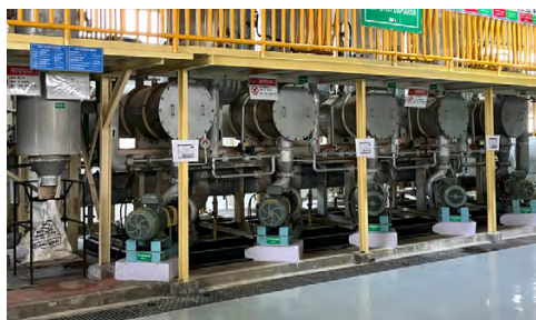
Wastewater recycling facility at the Tapukara Plant (India)
