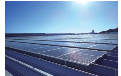
Saitama Factory Automobile Plant (2.0 MW)
