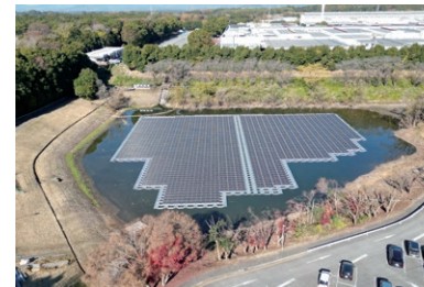
Kumamoto Factory (5.7 MW)
