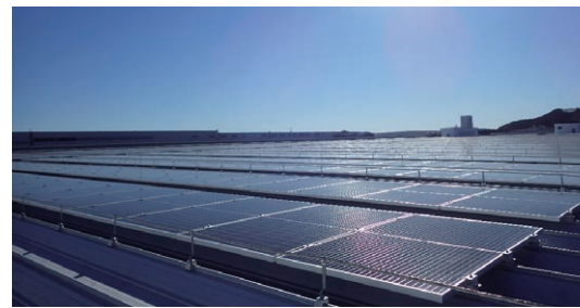
Saitama Factory's Yorii assembly plant (2.0 MW)
