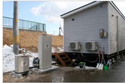
An MCHP1.0K2 gas engine cogeneration unit supplies power and hot water to a trailer house being used as a store for local specialty products and as a multipurpose space where volunteers care for elderly who live alone. A local NPO is orchestrating the two-and-a-half-year program.
