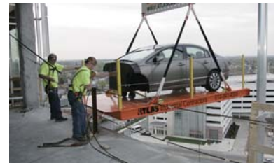
Moving a Civic with various rehabilitation-related modifications into the new hospital building
