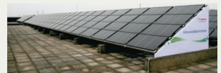
Rooftop solar panels at Dongfeng Honda
