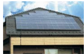
Installed solar array
