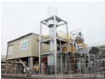
Natural gas cogeneration system (Kumamoto Factory)
