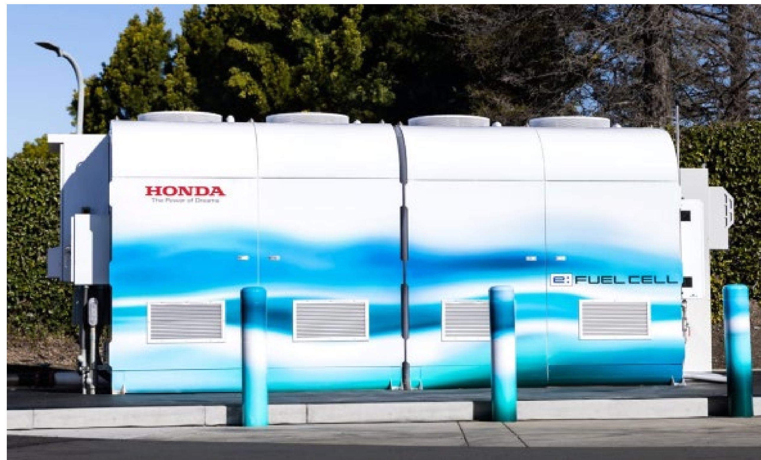
Installed in the premises of American Honda Motor Started in-house demonstration as emergency power generation for data center
