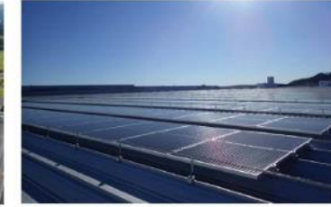
Saitama Factory's assembly plant (2.0 MW)
