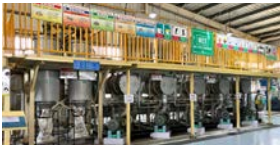
Water discharge recycling system at the Tapukara Plant in India
