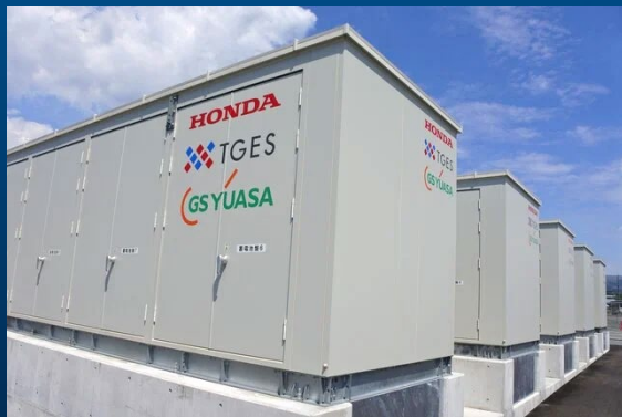
Lithium-ion storage battery facility (Container system)
