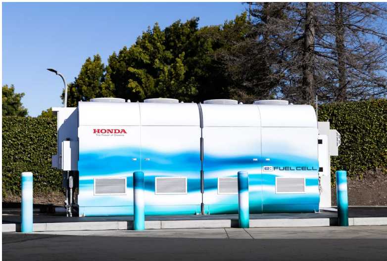
Honda's stationary fuel cell power station
